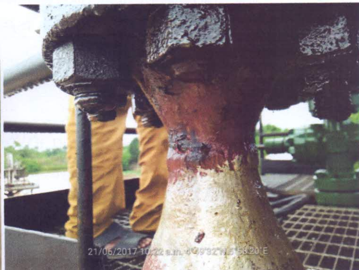
B: LEAK POINT
