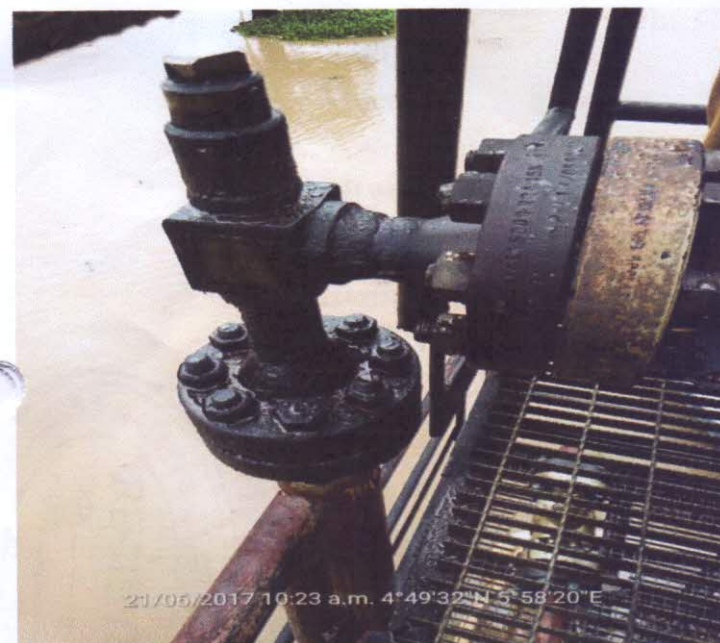
C: RUSTED BOLTS IMMEDIATELY ABOVE LEAK POINT
